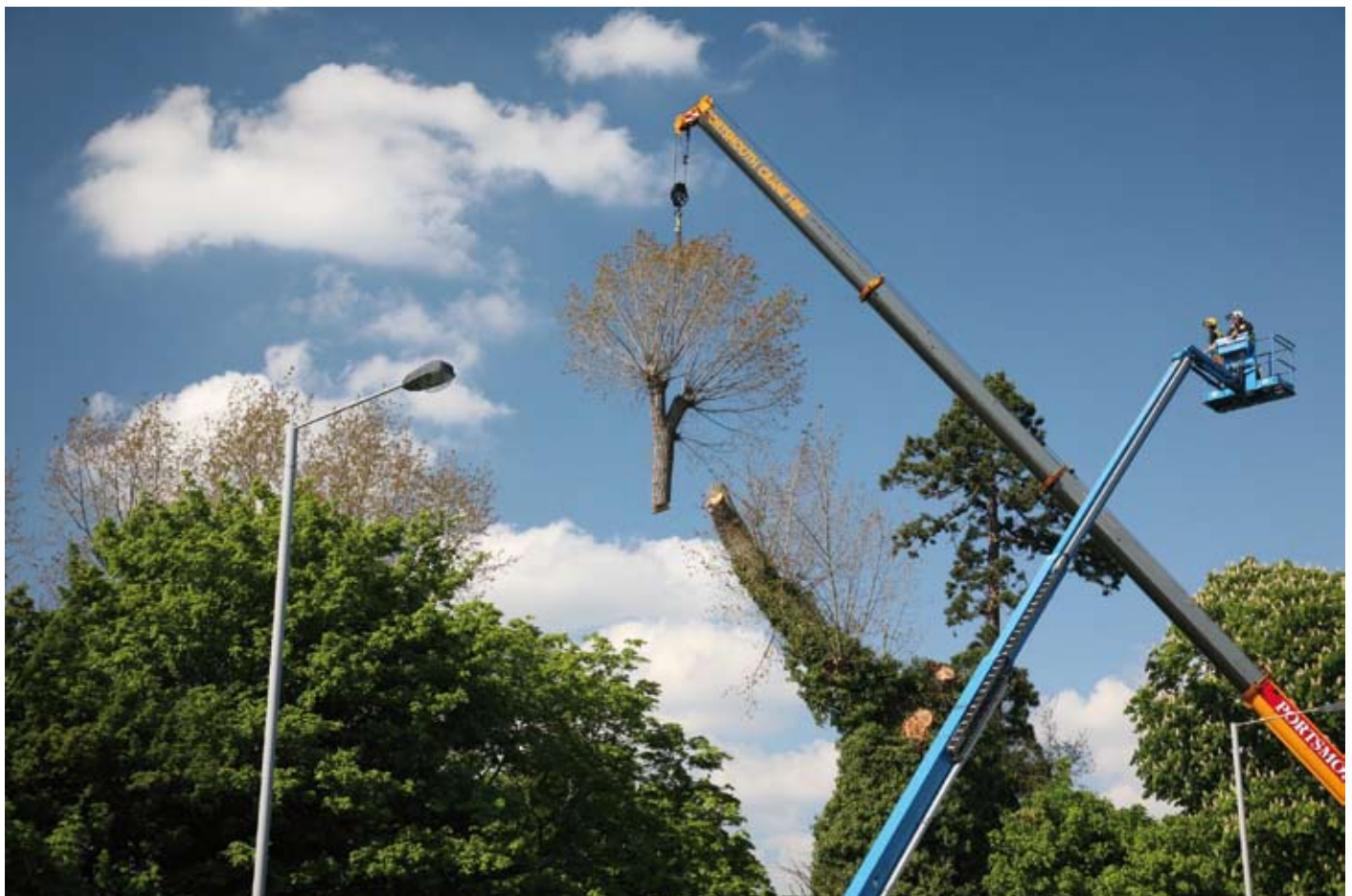
Crane and MEWP used to dismantle a Populus serotina, home to bats and with less than one-third residual wall, over a red route in London!
