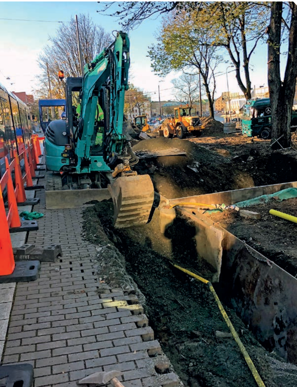
Figure 7: The proximity of regular rumbling trams took its toll on the structural integrity of the side walls of the excavated pit causing the tram platform to partially collapse and the tram stop had to be closed. (Photo: Hugo Loudon)
